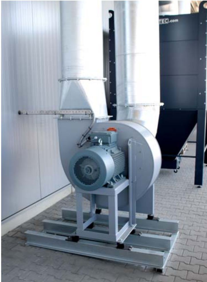
Radial blower MRG 18.5 kW connected to filter unit
