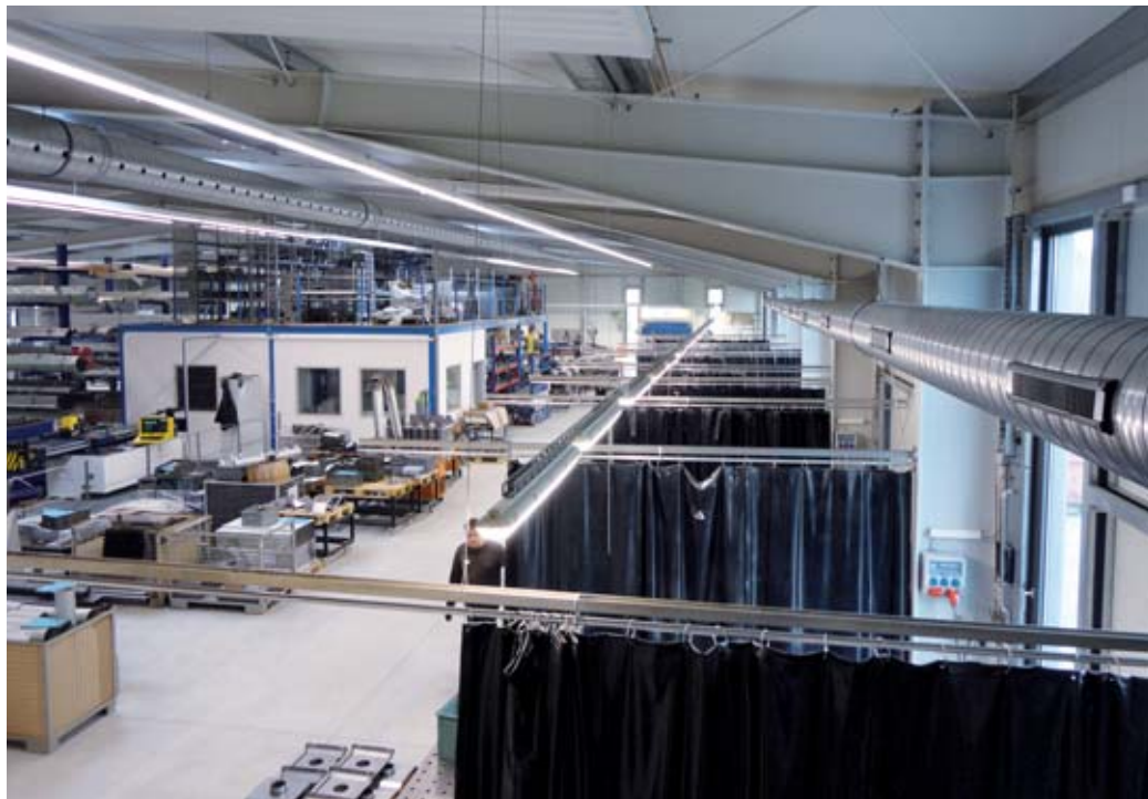
Pipe system for hall extraction
